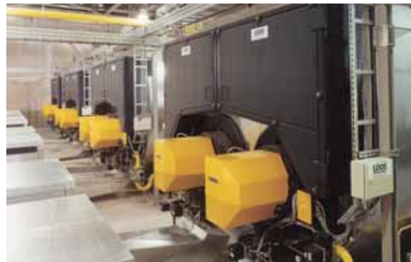
Four ZFR UNIVERSAL double flame tube boilers for producing saturated steam for parallel or single flame tube operation
