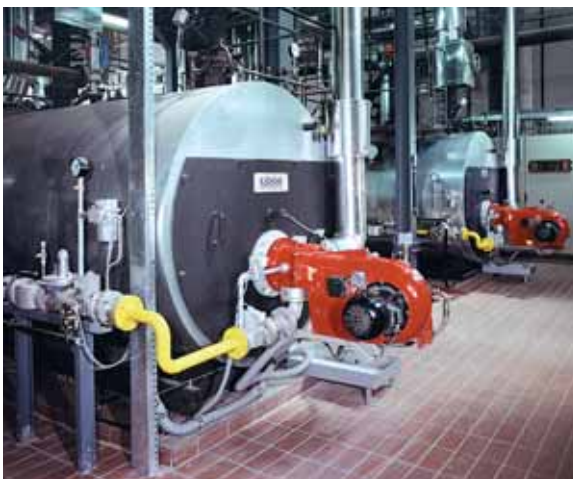
Two U-ND UNIVERSAL low-pressure steam boilers with modulating natural gas firing
