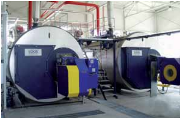
Two UNIVERSAL UL-S single-flue boilers for saturated steam, total system output 32,000 kg/h, pressure 10 bar
